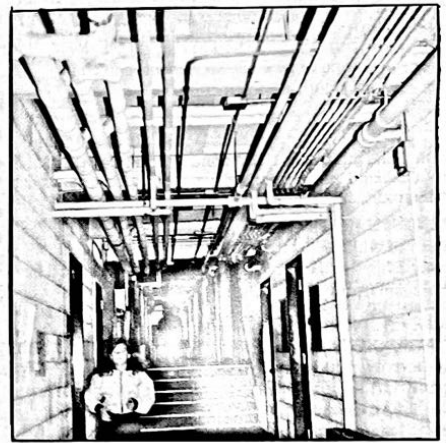
Middle School ceiling is lined with exposed heating pipes installed over 20 years ago to replace a failed heating system.
